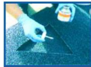
Apply some primer to all edges to act as a bonding agent
